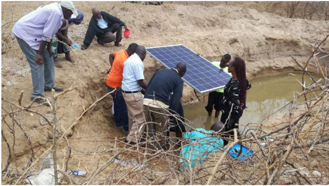
Officers from IFK, County government and service provider installing solar water pump during demonstration (Mwala Sub-County)
