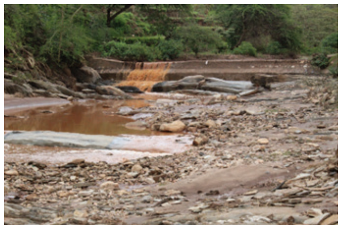
The effects of uncontrolled sand harvesting along Usiunene river, Kilome Sub County-Makueni county
